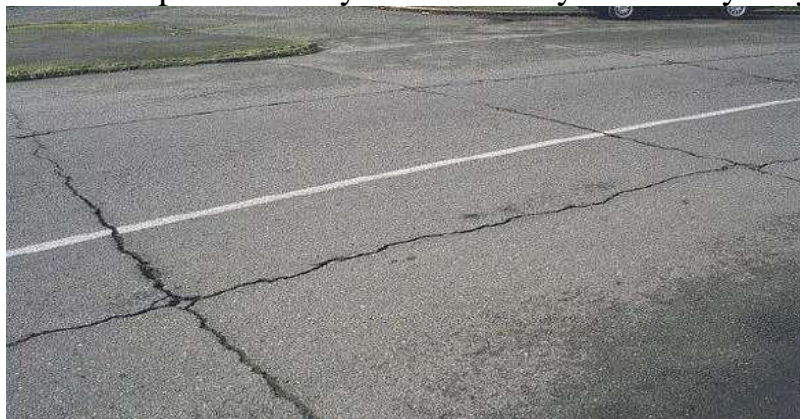
Fig. Joint Reflection Cracks
