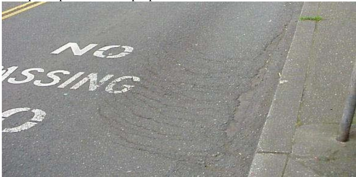
Fig. Slippage Cracks
