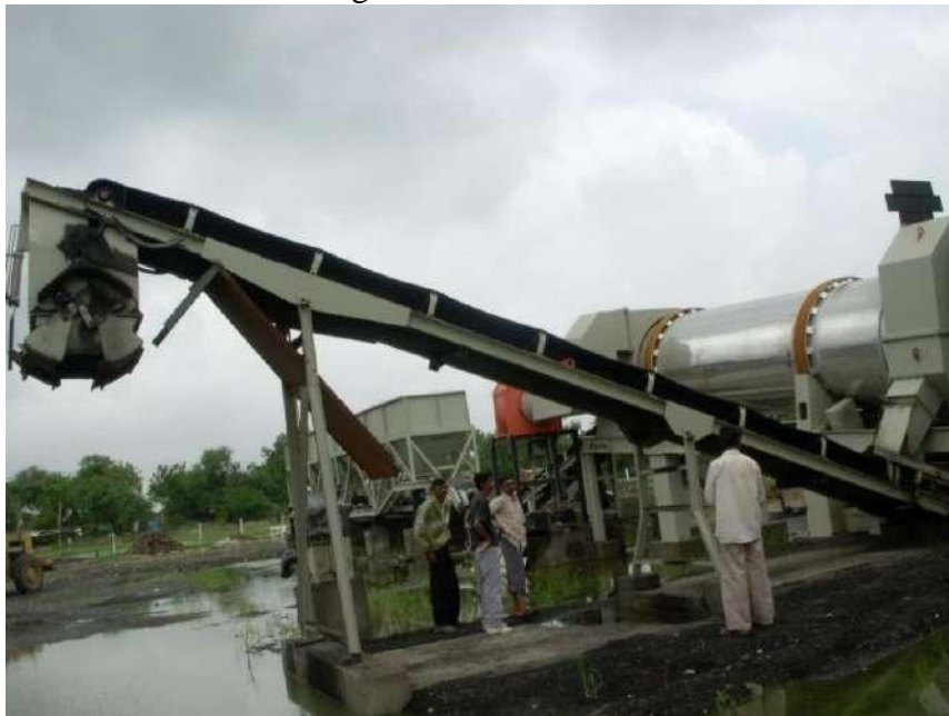
Fig. Load Out Conveyor
