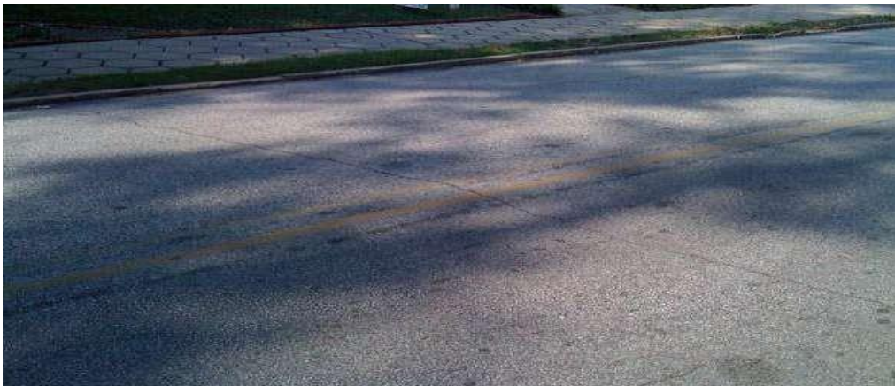
Fig. Transverse Cracking
