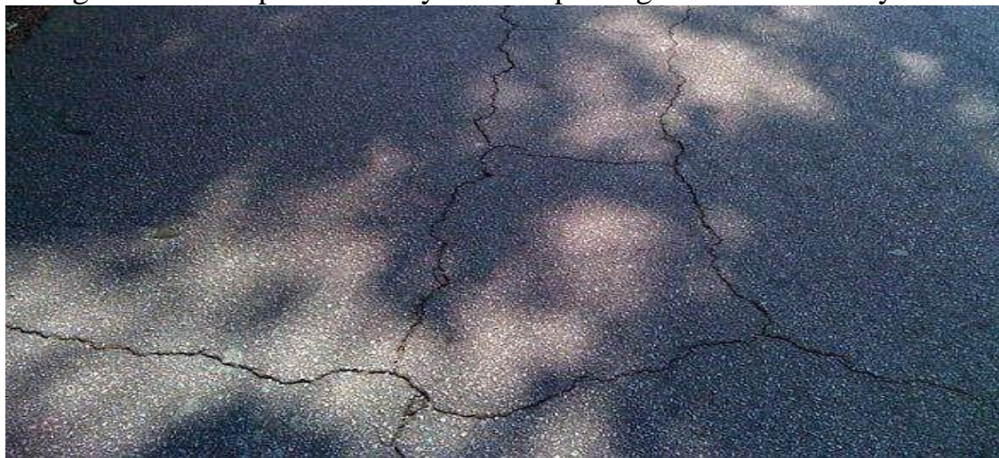
Fig. Block Cracking
