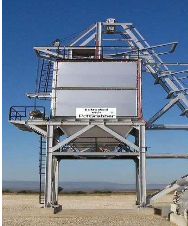
Fig.Hot mix storage silo
