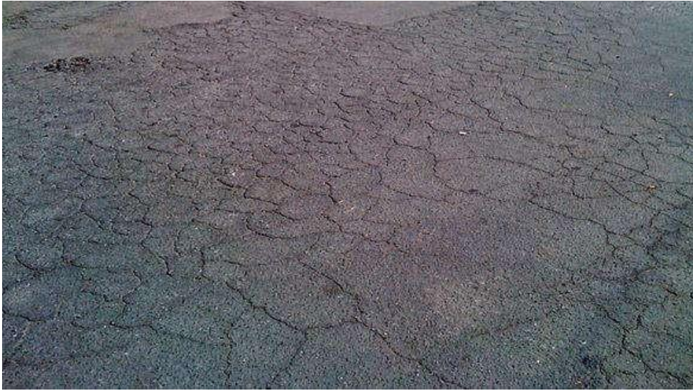
Fig. Alligator Cracking
